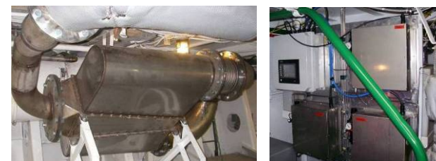
Compact SCR installation in M.V. Alcatraz Clipper
